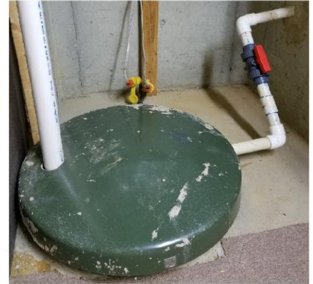
Top cover View of Grinder Pump in basement floor
